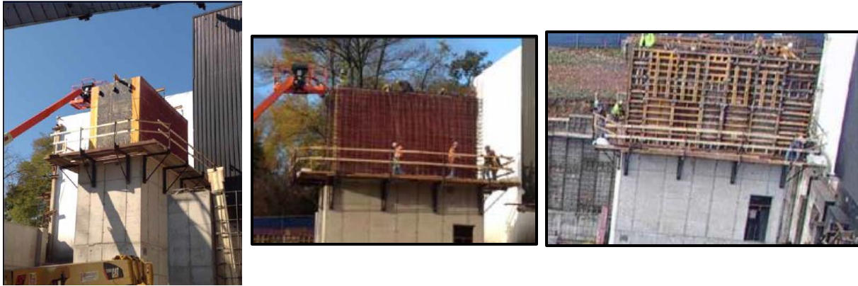
Figure 14 Installation Process for Stair Tower A. (From Left to Right) Installation of Interior Formwork, Installation of Rebar, and Installation of Exterior Formwork. This process is concluded with the concrete pour.
