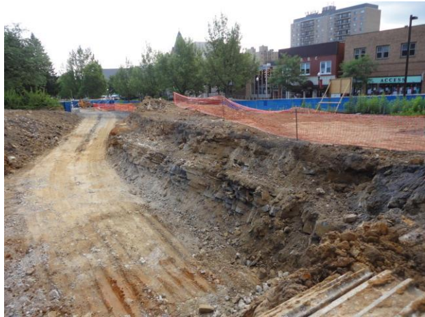
Figure 56 Sheared off Rock due to Blasting Utilization
