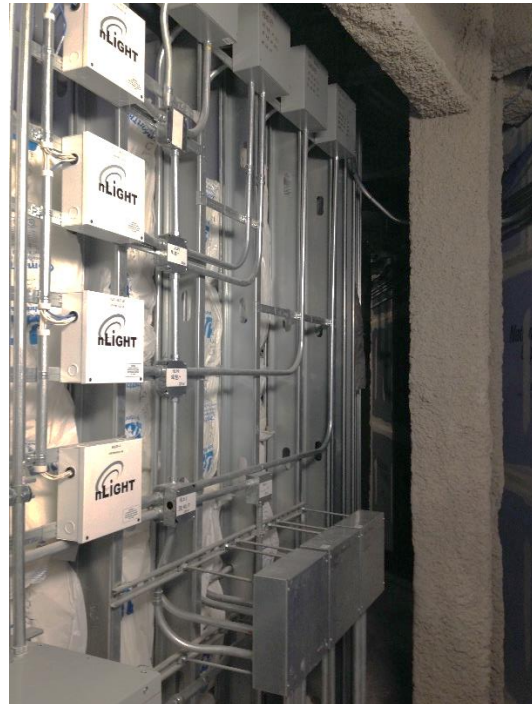
Figure 47 Return Air Plenum Space Utilized in a Wall at the Biobehavioral Health Building on Penn State's Campus
